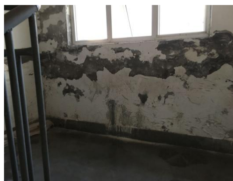
墙面渗水，墙皮脱落
