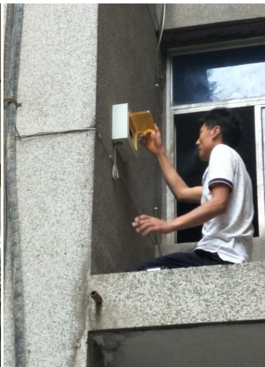
雁塔校区检修 15 号家属楼跳 闸情况
